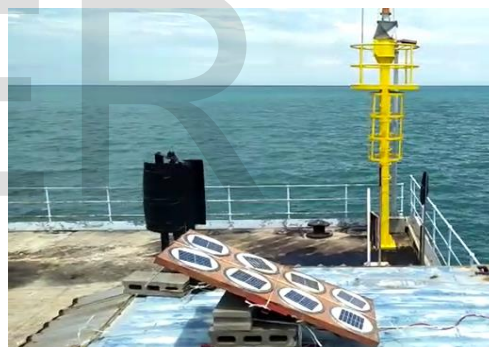
Figure 7. Installation of a hybrid wind solar system at the jetty of PLTU Rembang
